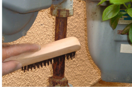
2. Wire brush so that the surface is free from loose rust, dirt and old, loose coating.
